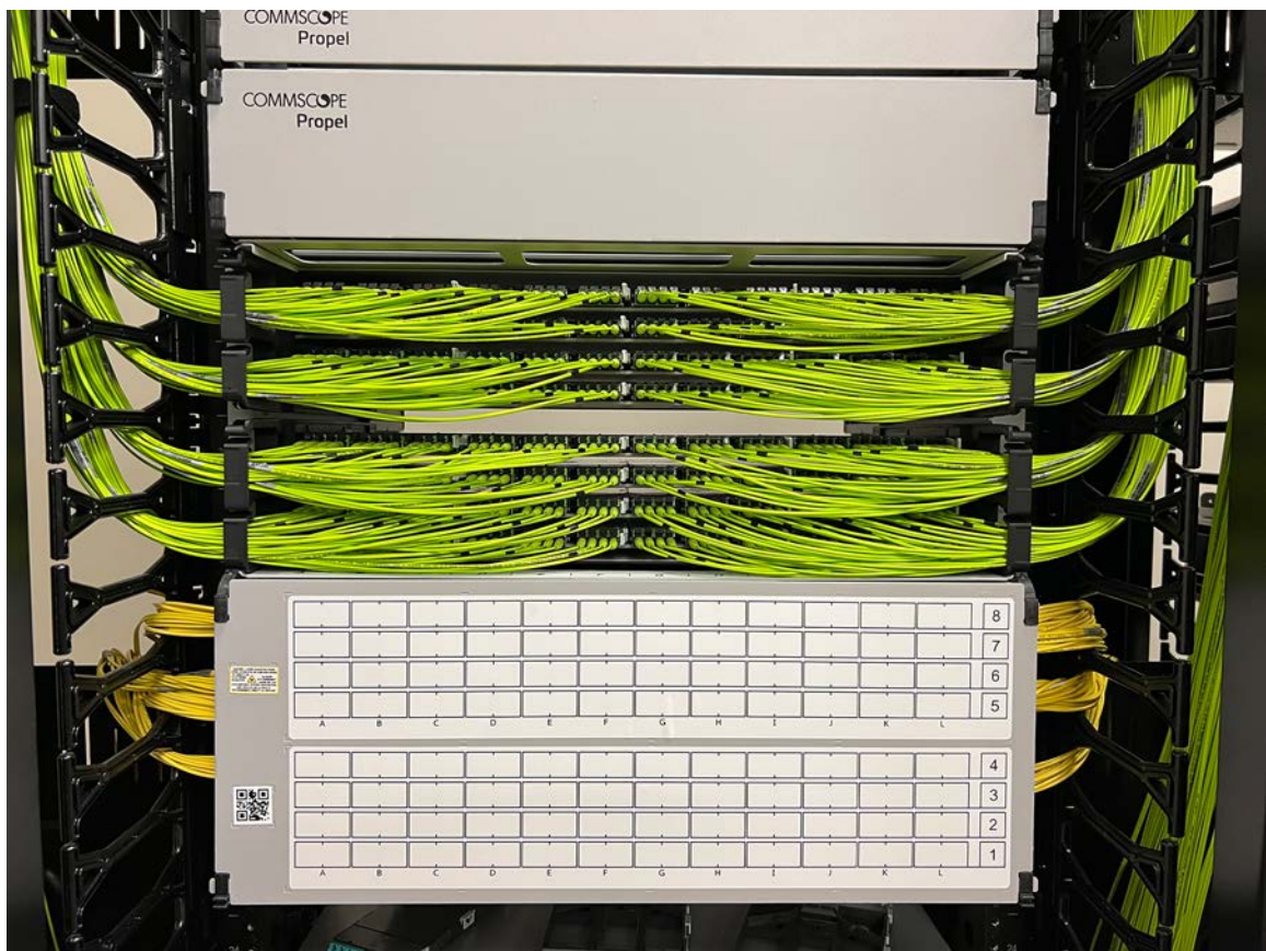
Figure 26. Patch Cords Fanned to Both Sides of a 4RU Fixed Panel
