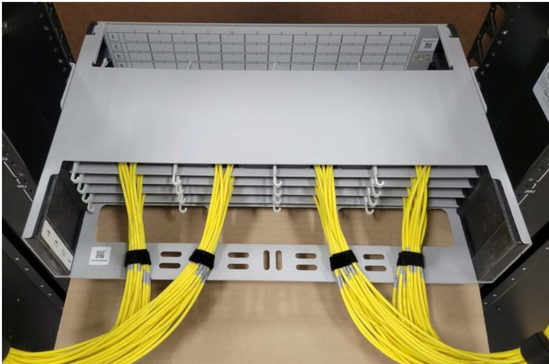
Figure 36. Securing Cables on a Fixed Open Panel
