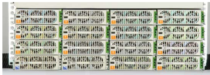
11.15: Converters and rectifiers occupying adjacent power shelf slots
