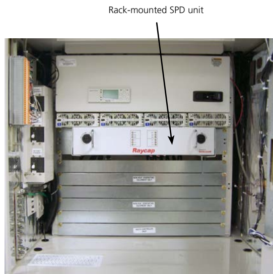
14.13: An SPD assembly mounted in a dc power and battery enclosure
